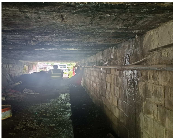
8#涵洞盖板钢筋锈蚀露筋
