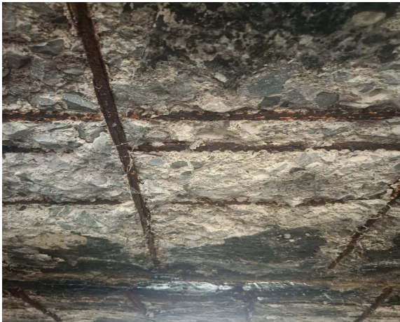
8#涵洞盖板钢筋锈蚀露筋
